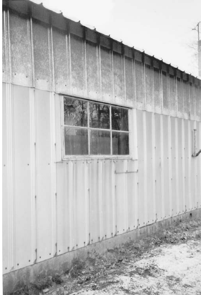
FIGURE 14.10 Rusting wall fasteners and window framing bleed through the paint.
